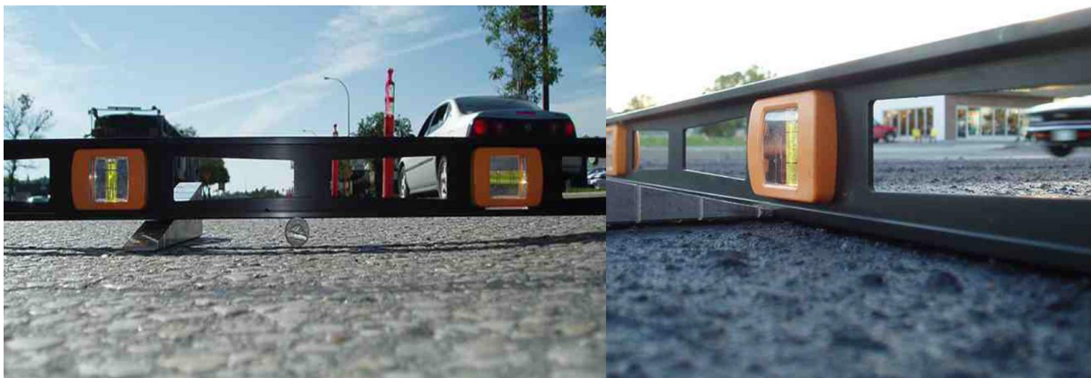
Figure 4. Micro surfacing used to fill wheel ruts: before (left photo) and after (right photo).
